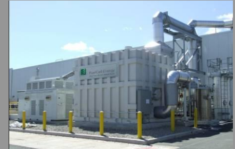
1.4 MW power plant
