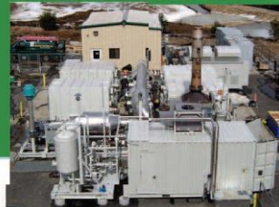
DFC1500MA 1.2 MW Fuel Cell Power System
