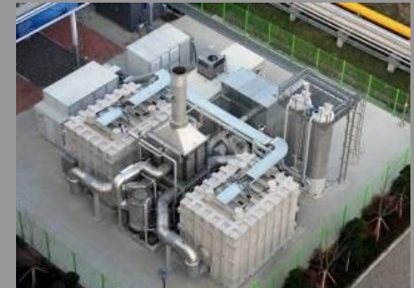
2.8 MW power plant
