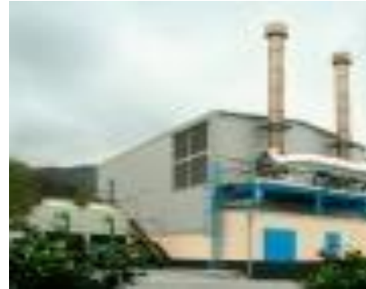
Gas Turbine CHP Plant
