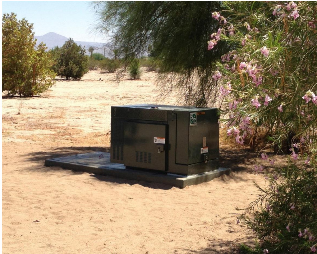
Photo Courtesy S&C Electric
