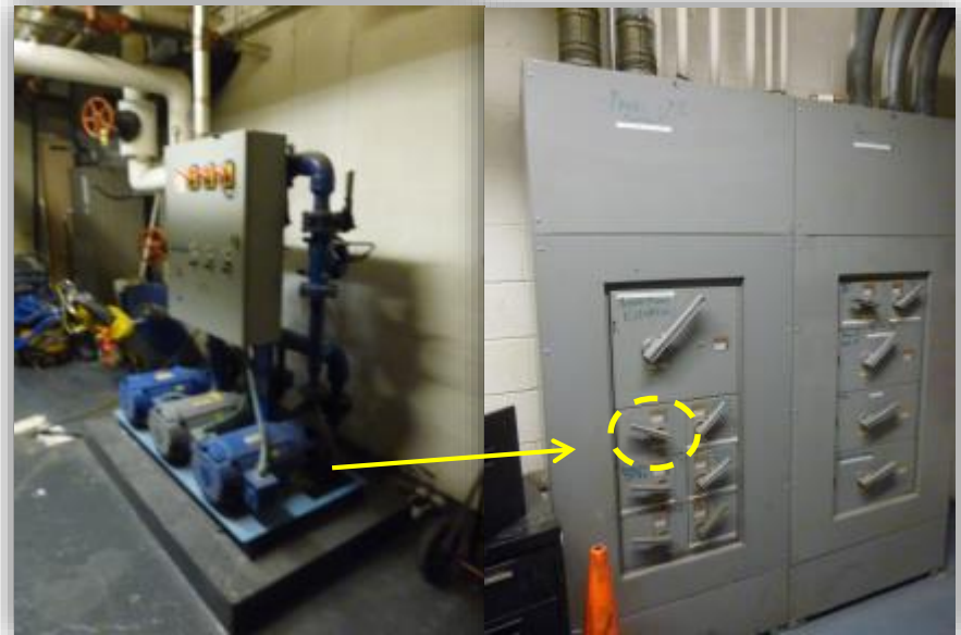
Water Booster Pumps
