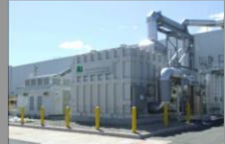
1.4 MW power plant
