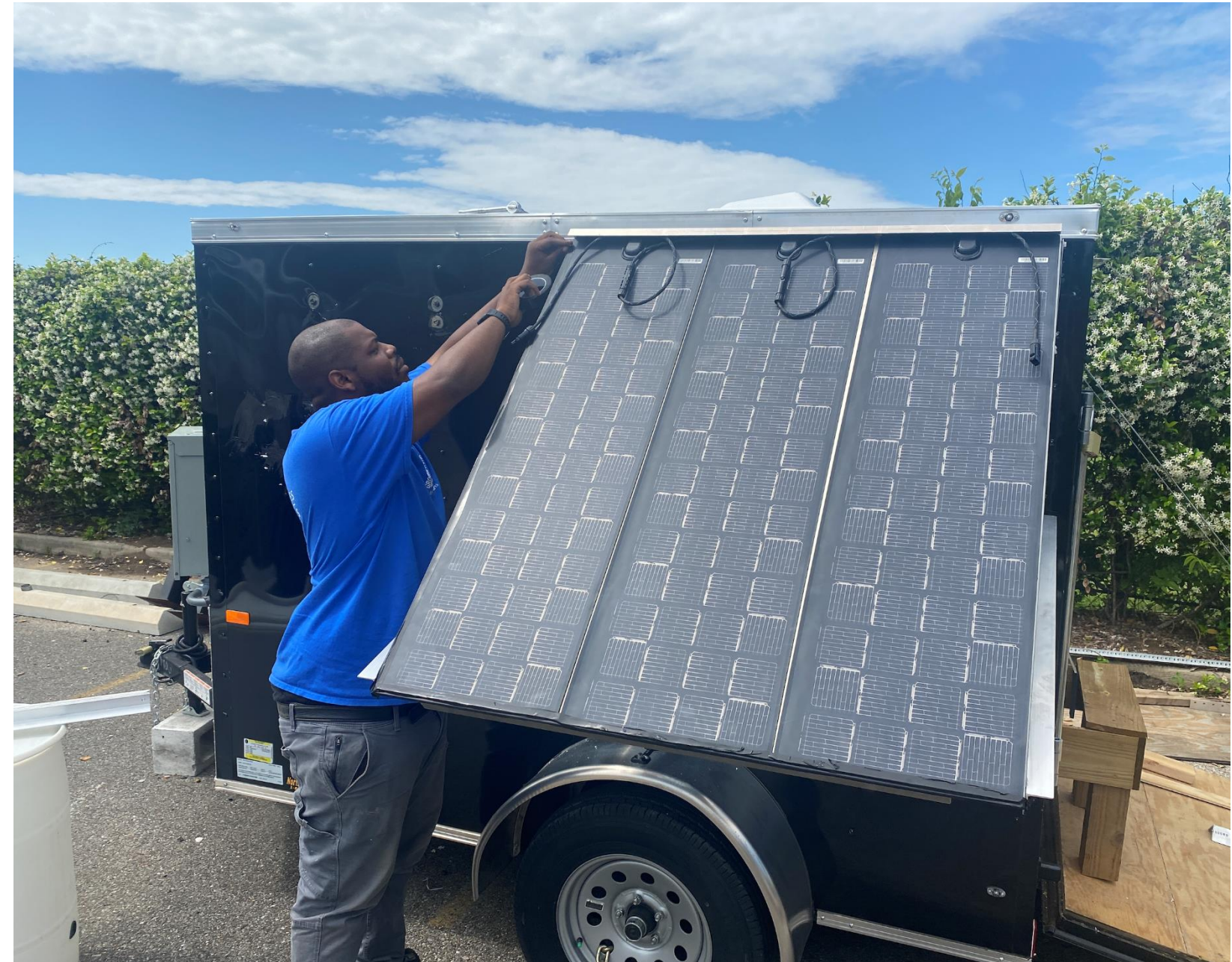
Installing a solar panel "wing" on a solar trailer. Credit: Footprint Project.
