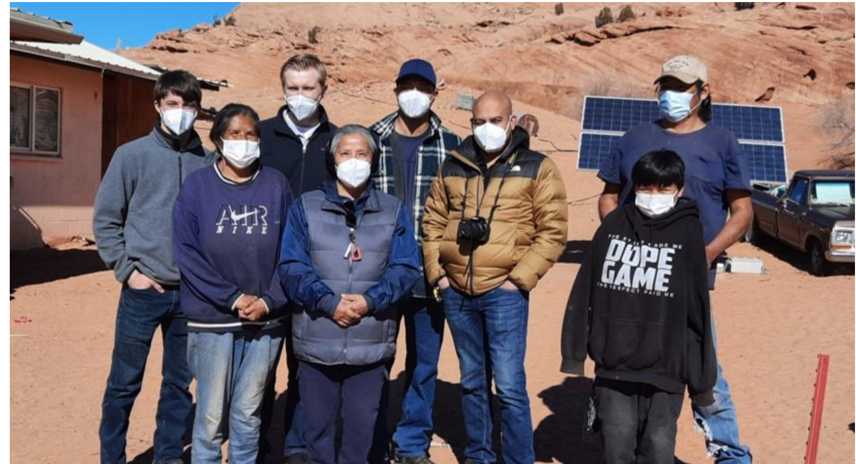
TAF engineering partners with Navajo Nation residents, installing solar+storage on their home. Credit: JPHB Solutions
