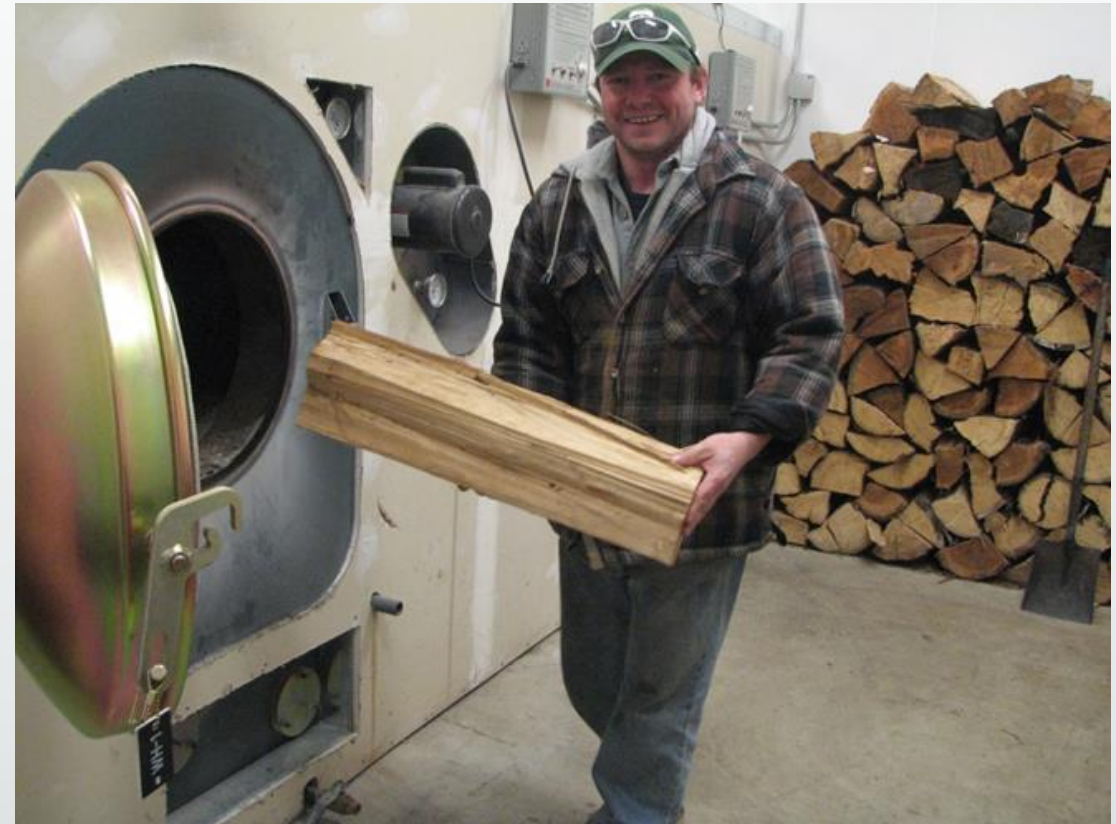
Coffman Cove School Garn boiler.
