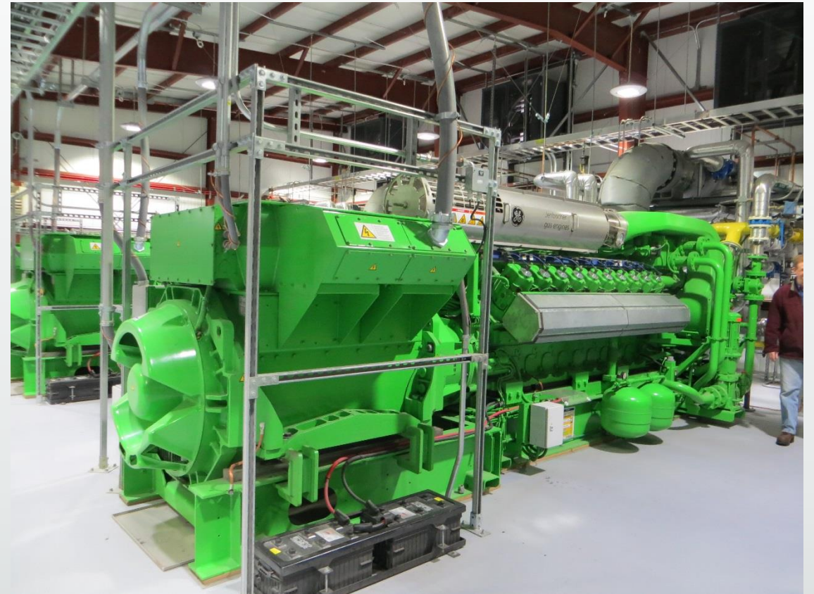
Anchorage Landfill Gas Project
