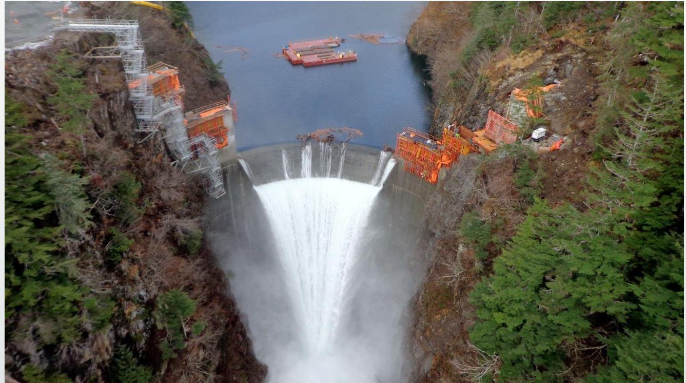
Blue Lake Hydro Expansion
