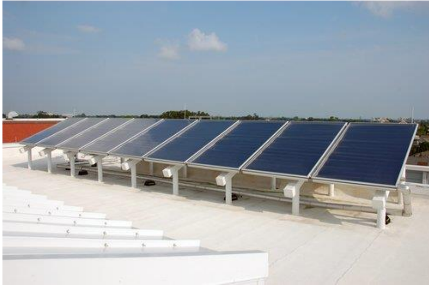
Collectors for solar water heating system on a school. NREL PIX 19690
