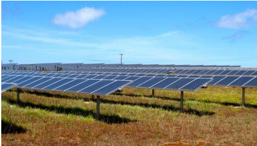
La Ola PV Plant in Hawaii. NREL PIX 19697
