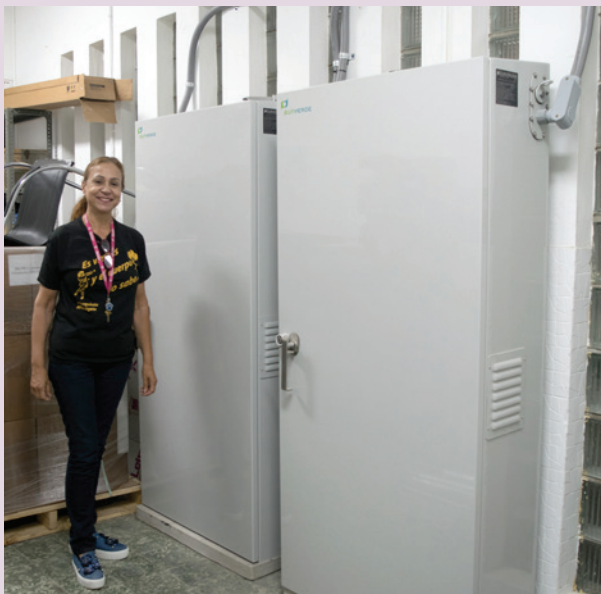
Battery storage system at a health clinic in Puerto Rico.
