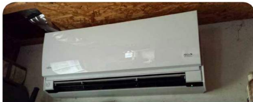
A ductless heat pump installed in a lobsterman's workshop on Islesford.
