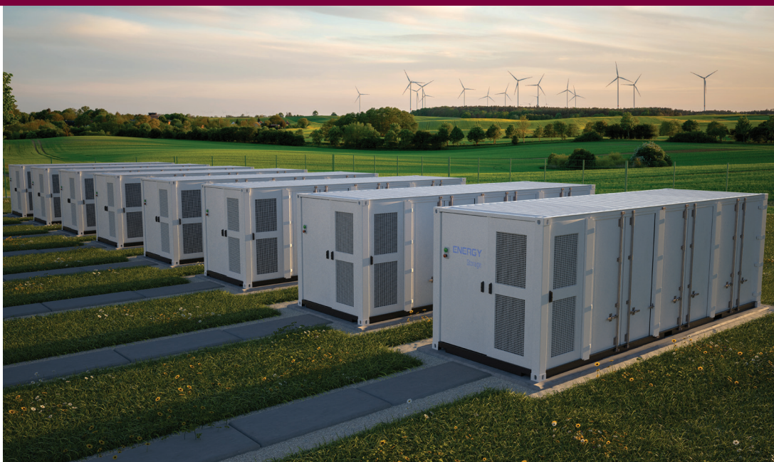
Battery energy storage systems, such as the utility-scale installation pictured here, can be paired with wind and solar.
