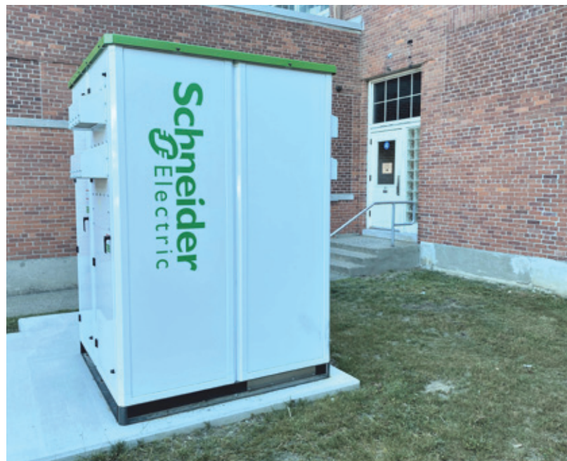
A 40-kW battery system installed at the Parsons Government Center in Milford, CT with funding from Connecticut Department of Energy and Environmental Protection's Microgrid Grant and Loan Program. This battery is part of a microgrid that includes a 400-kW combined-heat-and-power (CHP) generator. Facilities supported include City Hall, a middle school, a senior center and apartments.
