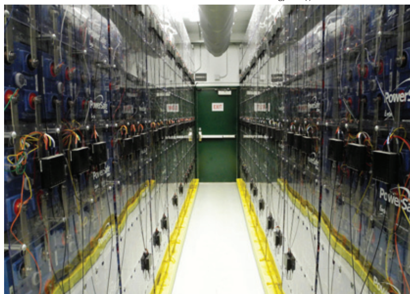
Interior of a lead acid battery container installed at the Stafford Hill Solar Farm and Microgrid in Rutland, VT. The Stafford Hill Solar Farm was one of the first microgrids in the US powered solely by solar and battery backup, with no other fuel source. It was supported by grants from Vermont Department of Public Service and US DOE Office of Electricity, as well as by technical support from Sandia National Laboratories and Clean Energy States Alliance.
