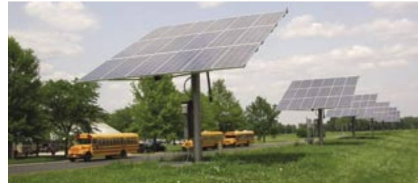
This 10-kw PV array at a vocational high school in Illinois was installed with support from the Illinois Clean Energy Community Foundation.
