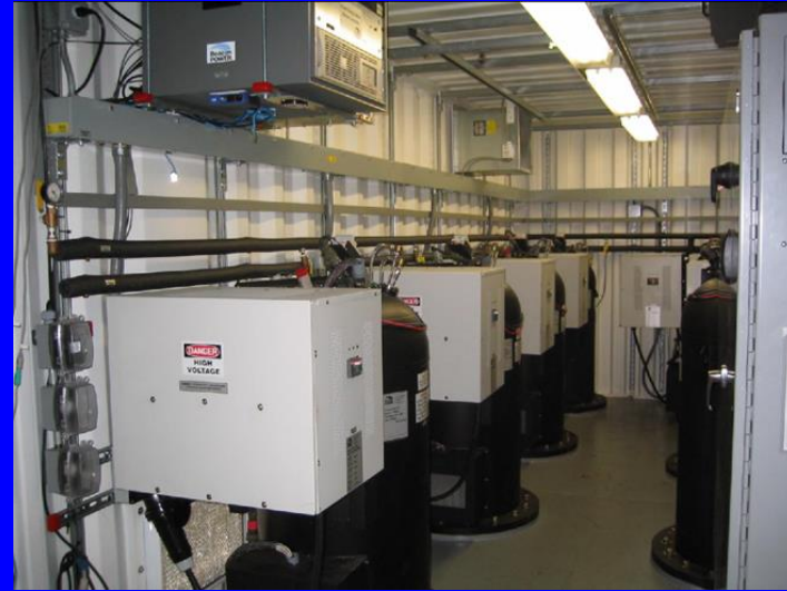
Containerized 7 Flywheel System
