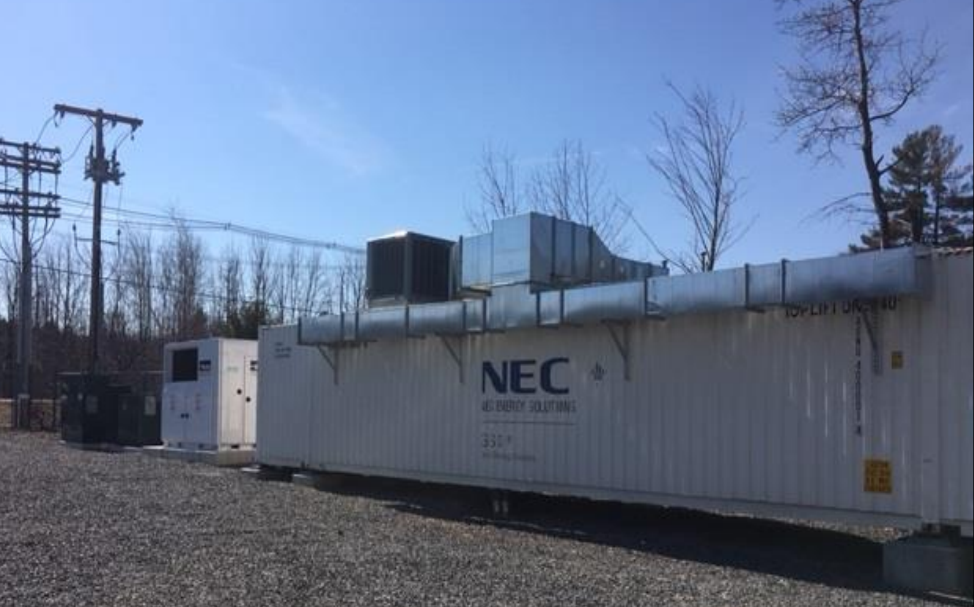
Sterling 2MW / 3.9 MWhr Battery Storage Project
