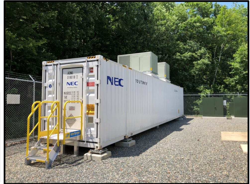
NEC Battery Storage Container & Step-up Transformers
