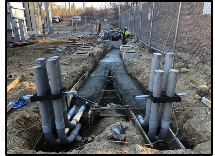
Conduits for DC Cables to the Battery Container | 10
