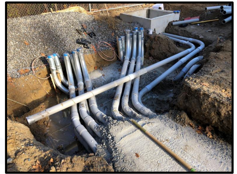
Conduits to the Step-up Transformers
