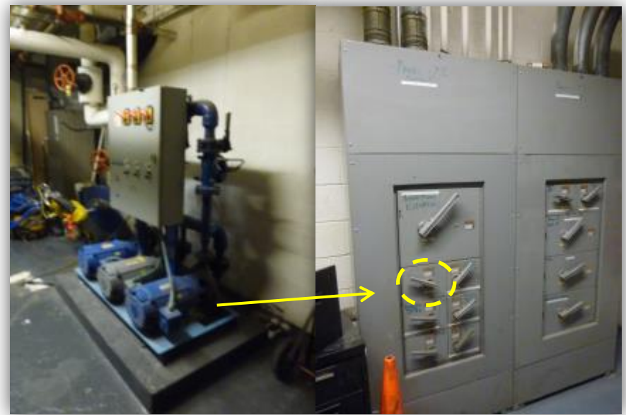
Water Booster Pumps
