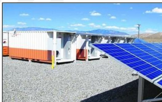
500-kW/1-MWh Adv LA: Time-shifting 900-kWh Adv Carbon Valve-regulated: PV Smoothing
