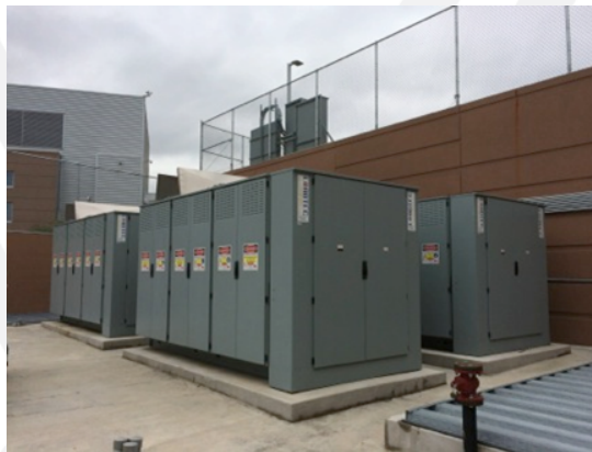
1 MVA RLC Load Bank
