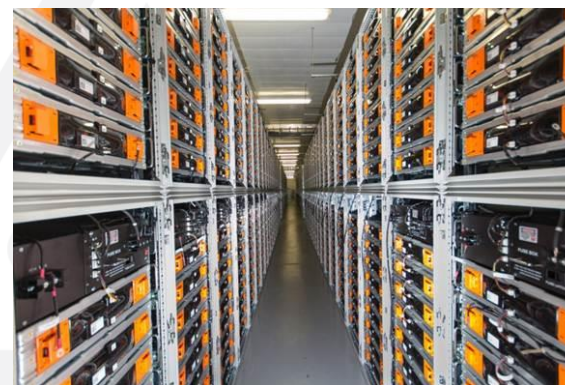
Tehachapi Wind Energy Storage Project - Southern California Edison Lithium-Ion Battery 8-MW / 4 hour duration
