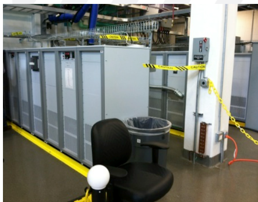
1.5 MVA PV Simulator
