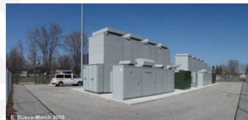
Sodium Sulfur Battery 2 MW / 8 hour
