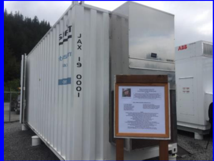
1 MW / 1 hr Li-ion Storage
