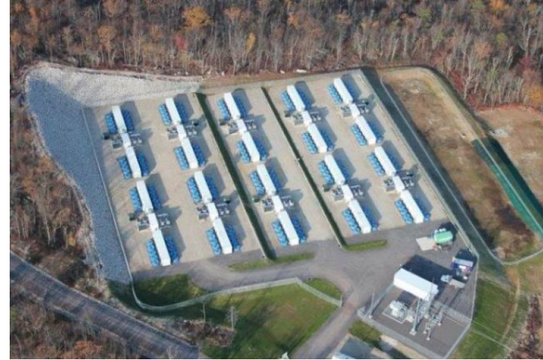
20 MW, 5 MWh Beacon flywheel plant at Hazle Township, Pennsylvania
