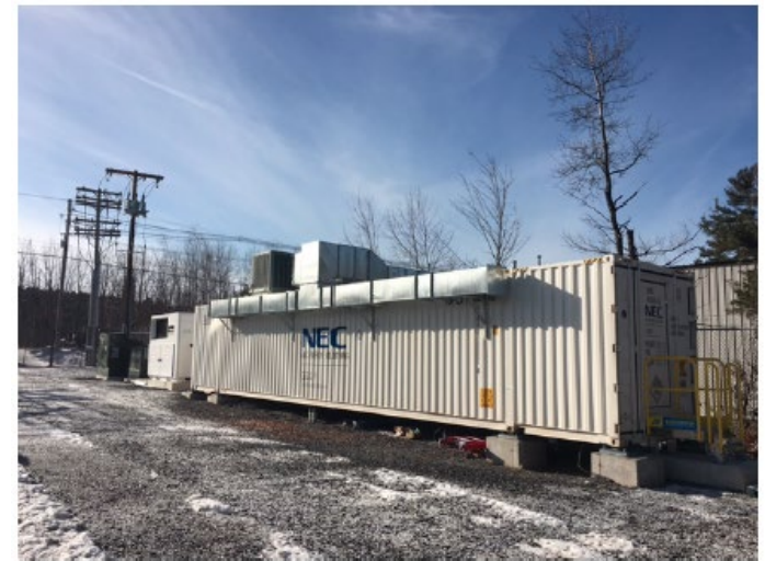
Sterling Municipal Light Department 2 MW, 3.9 MWh system
