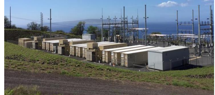
Standard containerized GSS ® grid storage solution
