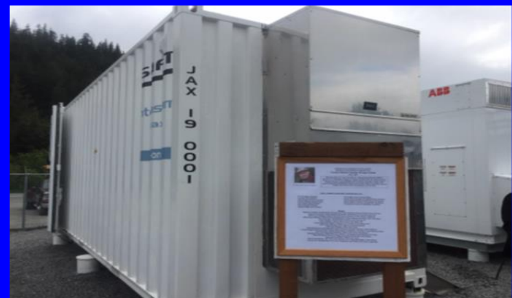
1 MW / 1 hr Li-ion Storage, Saft
