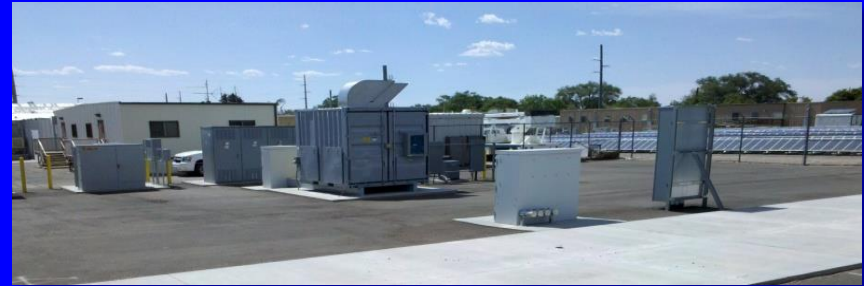
Energy Storage Test Pad (ESTP)
