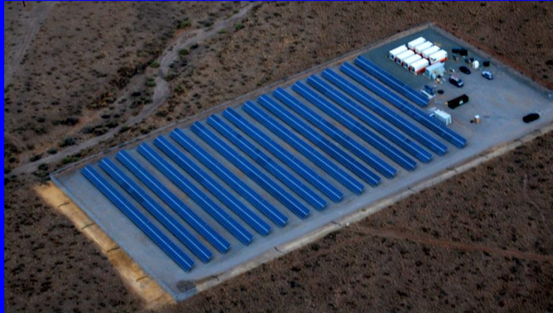
2011, NM: 500kW, 2.5MWh with PV
