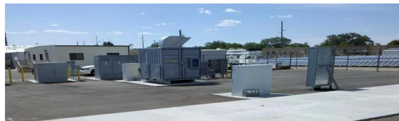
Energy Storage Test Pad (ESTP)
