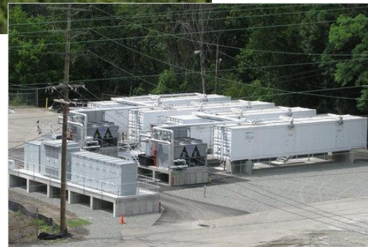
8 MW Li-ion battery system in NYISO
