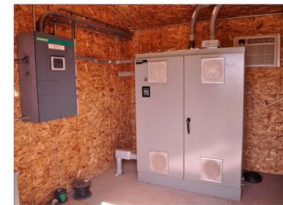
200 HP MOTOR STARTING VFD & 100 HP REGENERATION VFD WITH LOCAL CONTROL PANEL.
