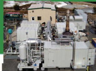
DFC1500MA 1.2 MW Fuel Cell Power System
