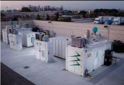
600 kW plant at a food processor
