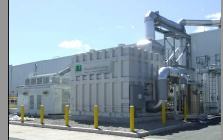
1.4 MW power plant
