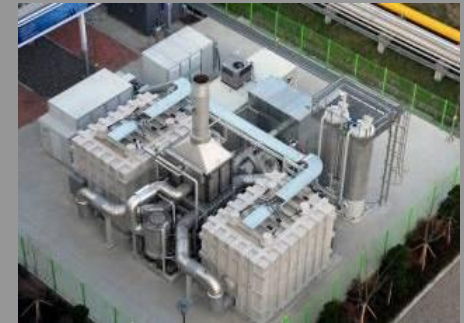
2.8 MW power plant
