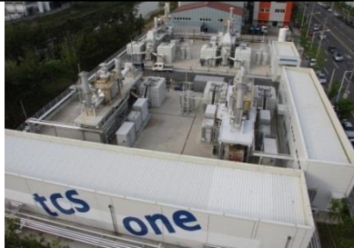
11.2 MW plant – World's largest operating fuel cell park
