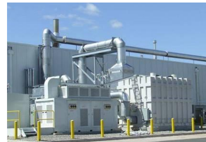
DFC1500 One 4-Stack Module 1.4 MW
