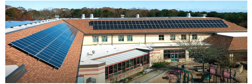
Oak Bluffs Elementary School Roof & BESS
