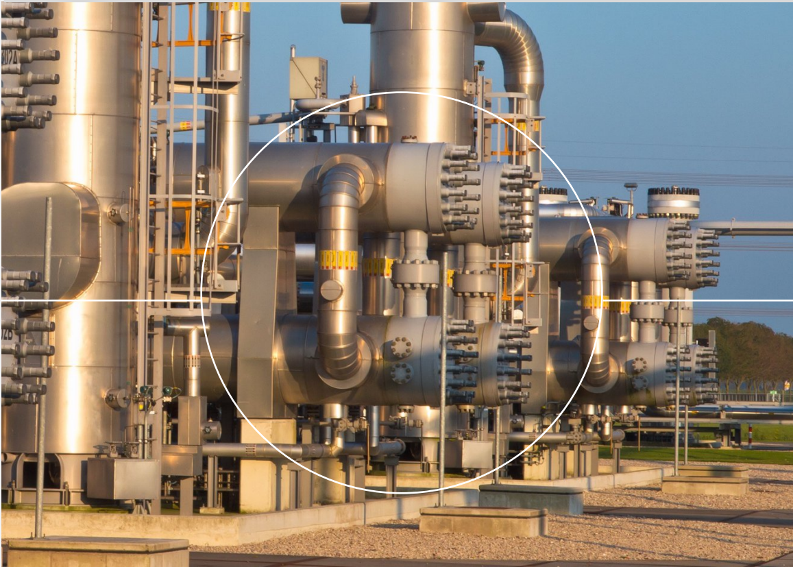
CONVENTIONAL INDUSTRIAL EQUIPMENT
