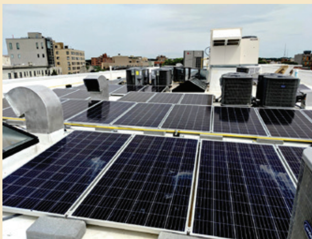
Solar array on Maycroft Apartments. Source: New Partners Community Solar.
