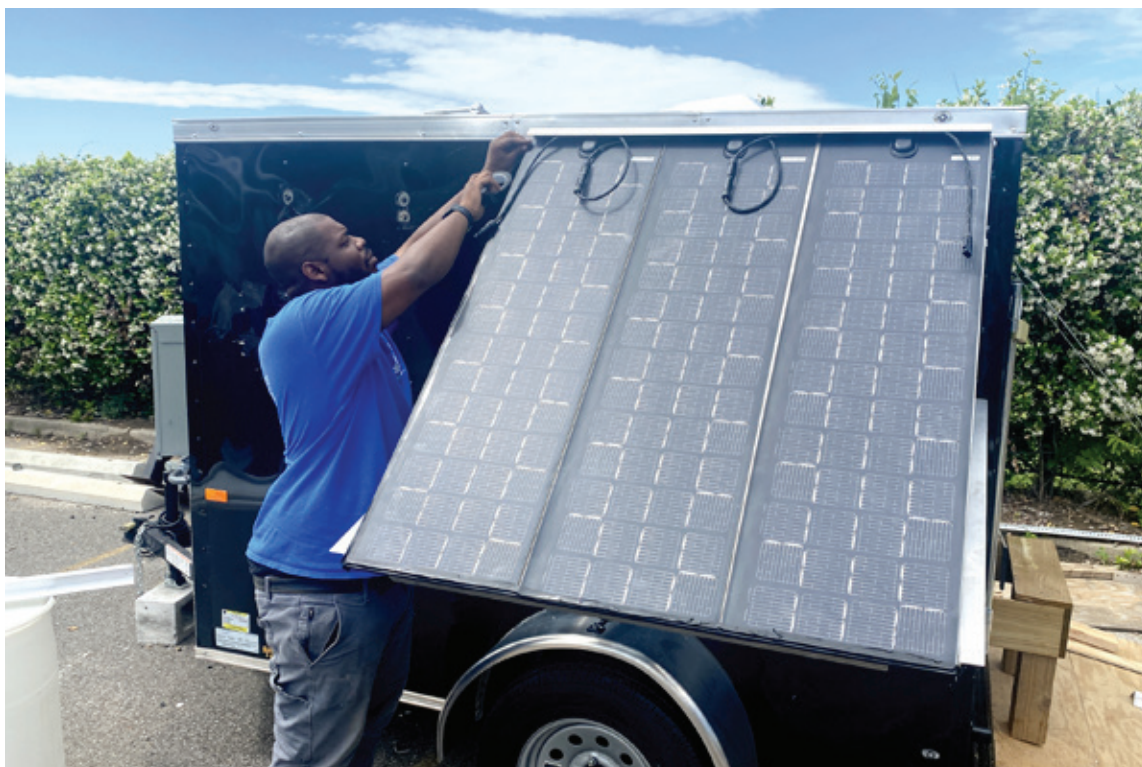
Willie Jones installing a solar panel “wing” on a prototype solar trailer “Bee” on the Net 2 Gentilly “Beehive.” Source: Footprint Project
