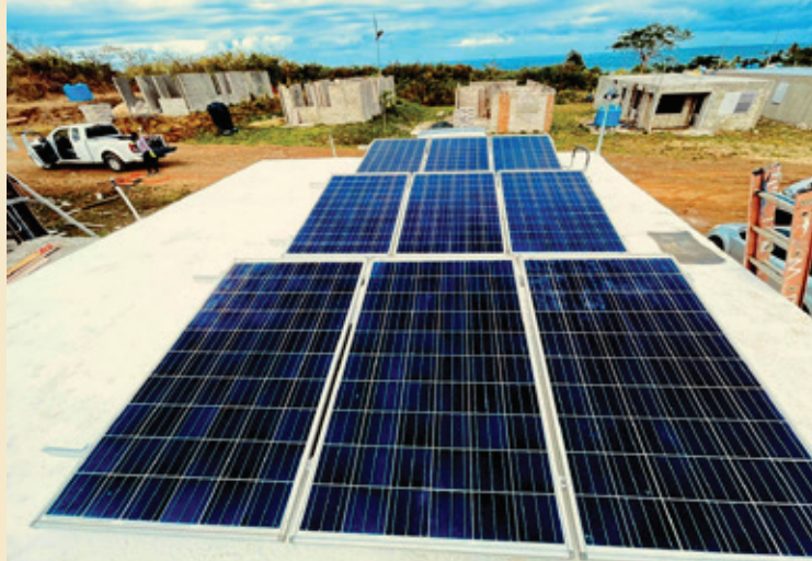
Rooftop solar installed in Vieques, Puerto Rico.
