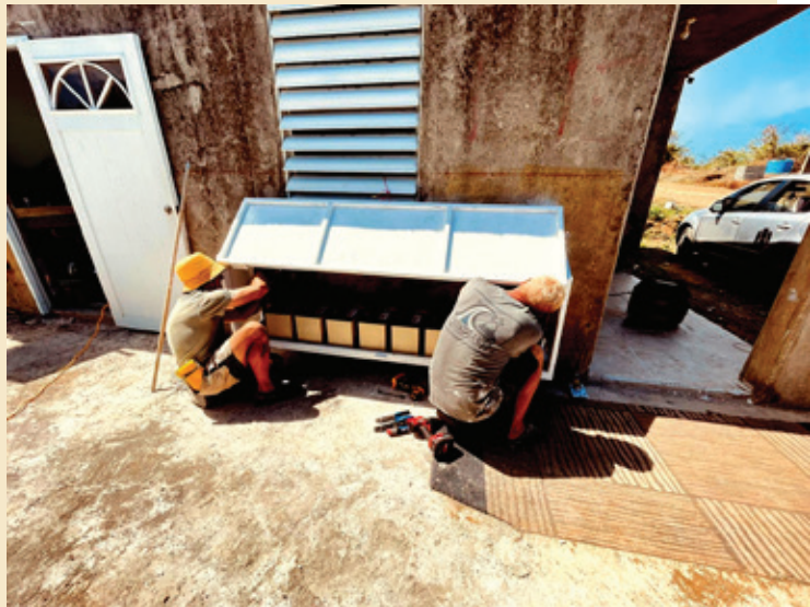
Battery installed in Vieques, Puerto Rico
