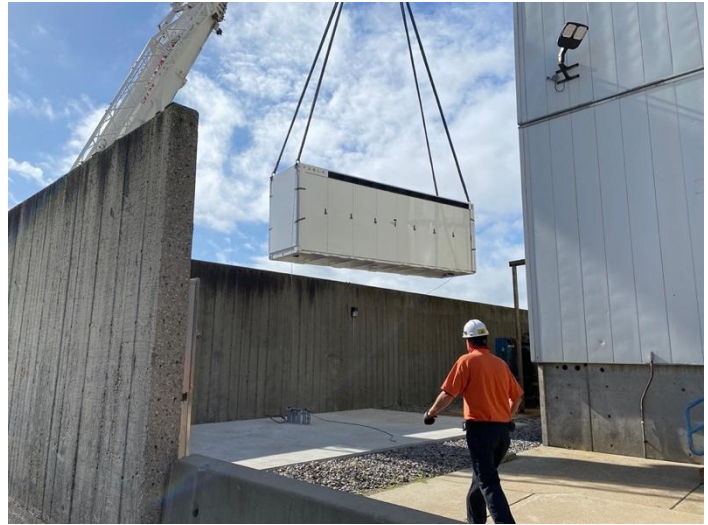
Battery being installed at Boston Medical Center. Source: Boston Medical Center
