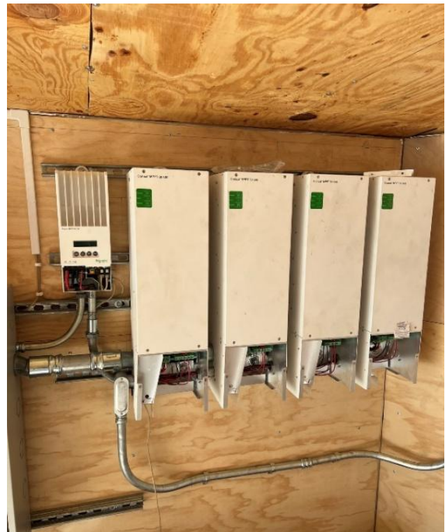
Four battery storage units and the solar inverter, located inside the Queen Bee semi-permanent trailer. (Credit: Groundworks New Orleans)
