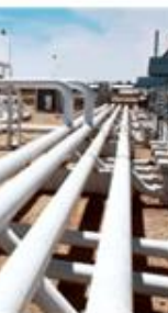
Natural Gas Pipeline Injection
