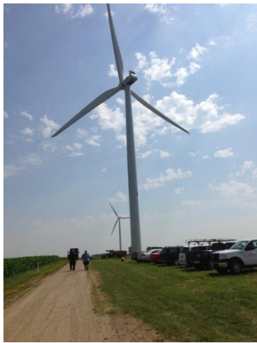
Onsite wind power
