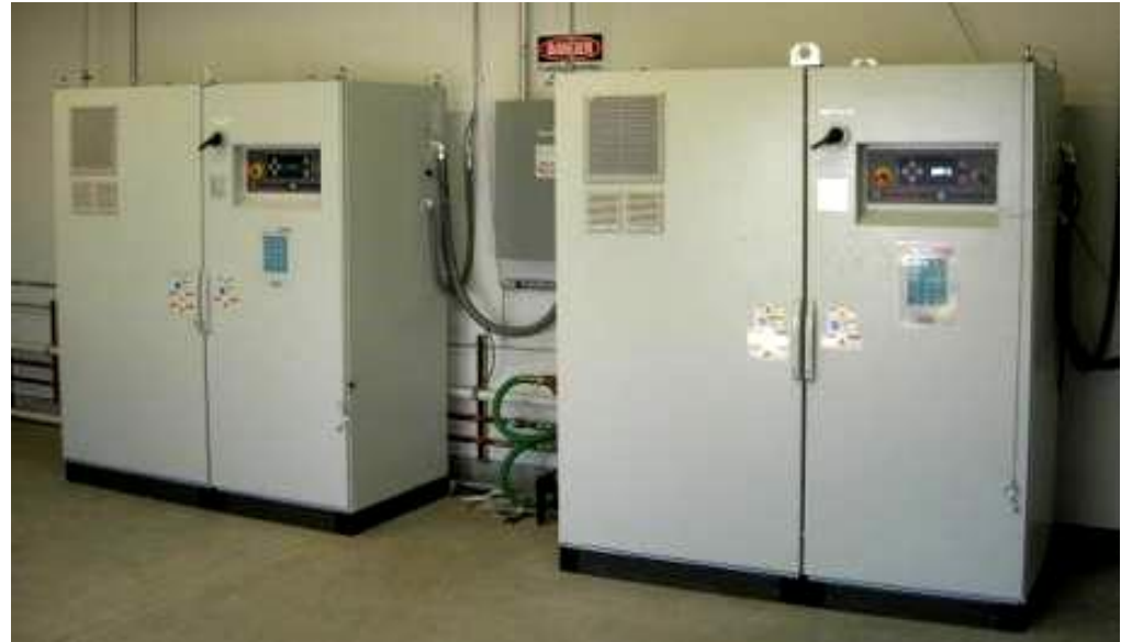
H6M Electrolyzers at Synthetic Energy
