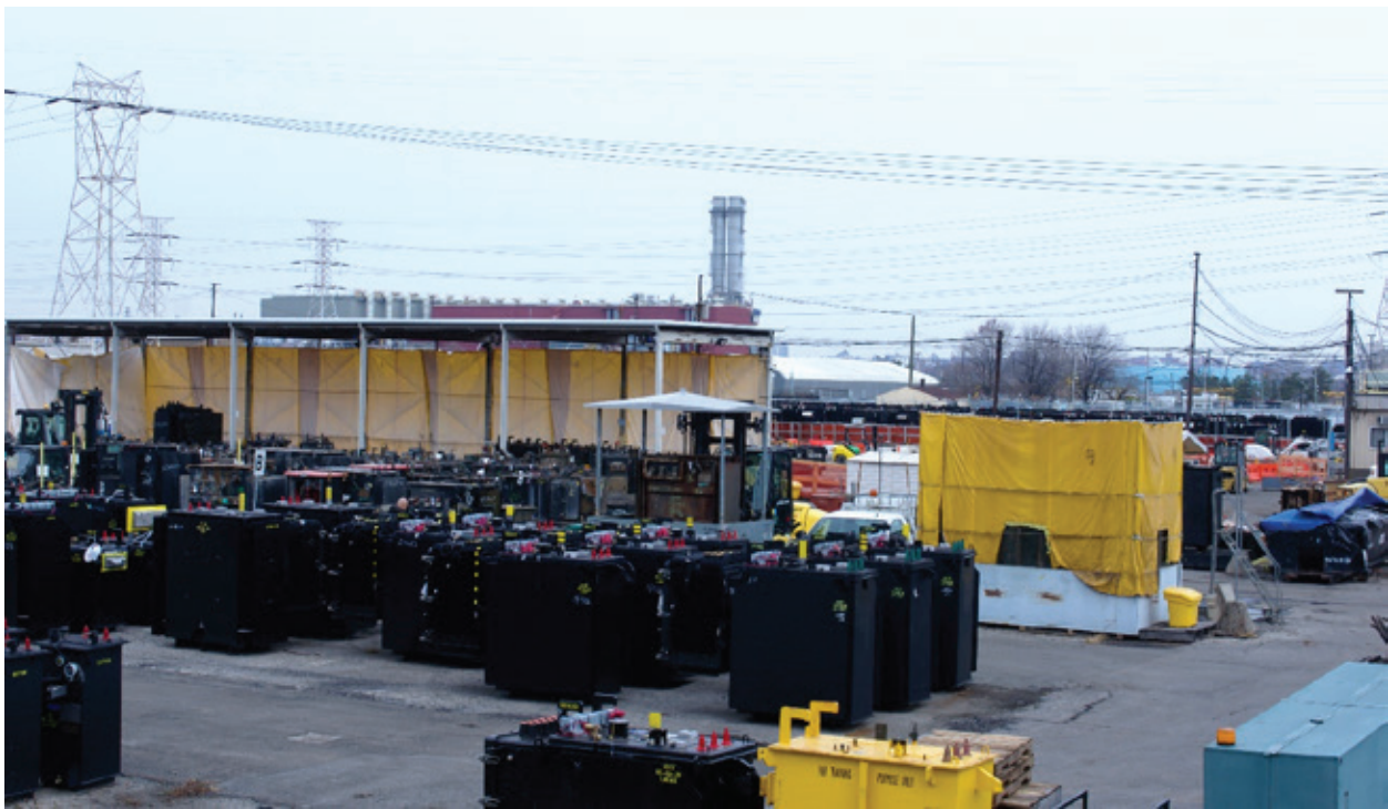
East River Energy Storage Project being built at the former site of the Charles Poletti power plant in Astoria, Queens. PHOTO: SEBASTIAN BAEZ/UPROSE
